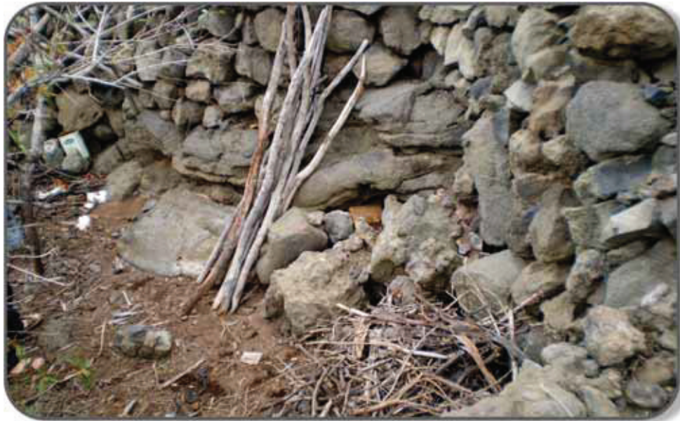
At the footstep of one of the Icod pyramids, there exists volcanic rock used as a foundation with the potential entrance. No excavation has been performed so far.
