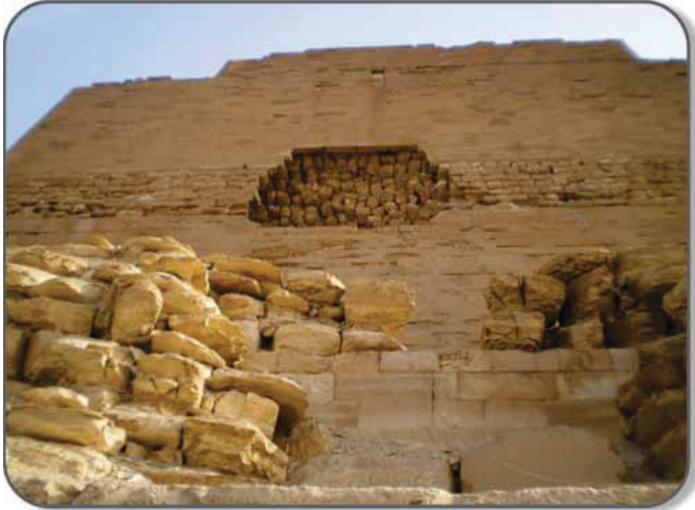
Damaged sections of the outer layer of the pyramid in Meidum
