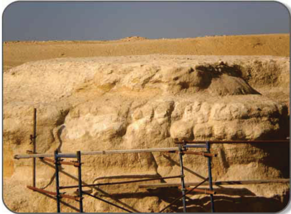
Apparent vertical erosion of the Sphinx; reconstruction will conceal important evidence of exceptional age of Sphinx.
